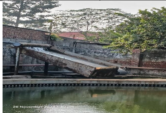
Photo 7: Secondary Clarifier & Hill screen
