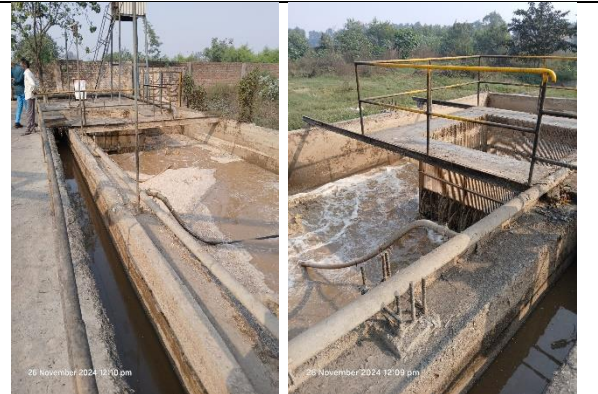
Photo 2: Equalization tank (Unit-1 & 2)
