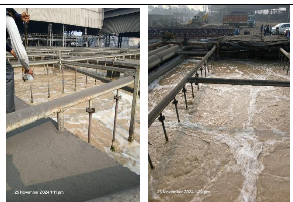
Photo 4: Aeration Tank (Unit-1 & 2)
