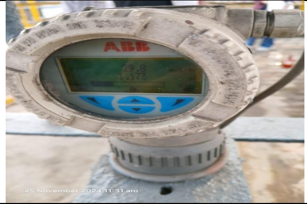
Photo 10: ETP outlet flow meter
