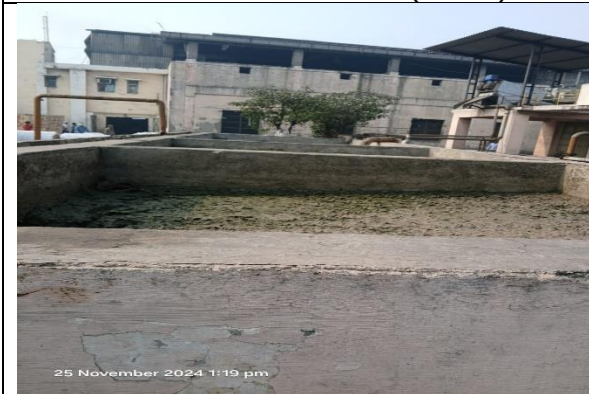
Photo 9: Sludge drying beds
