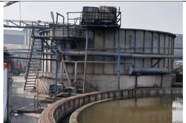
Photo 4: Sedicell & Primary Clarifier
