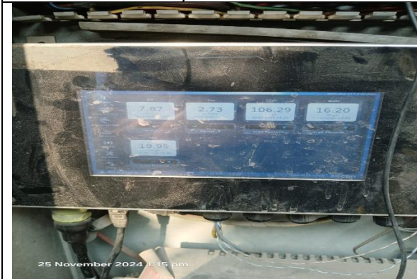
Photo 7: OCEMS at ETP outlet (unit-1)
