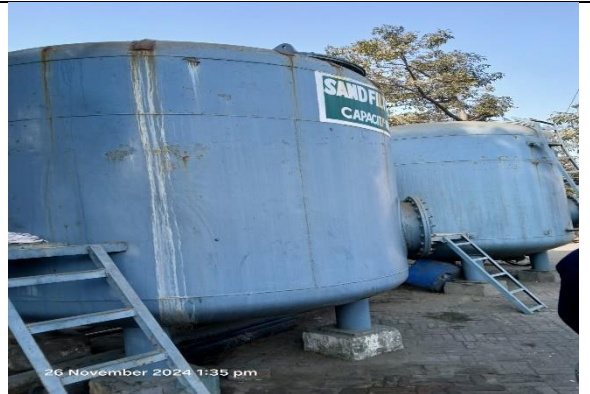
Photo 8: Tertiary filtration units
