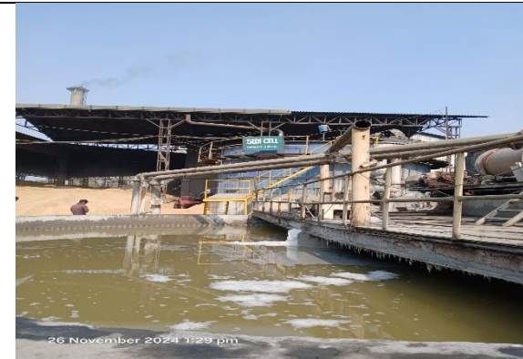
Photo 5: Sedicell & Primary Clarifier
