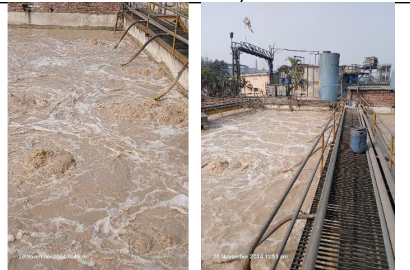
Photo 6: Aeration Tank (Unit-1 & 2)
