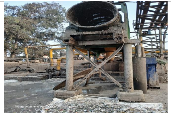
Photo 2: B2 thickener (plastic separation from effluent)
