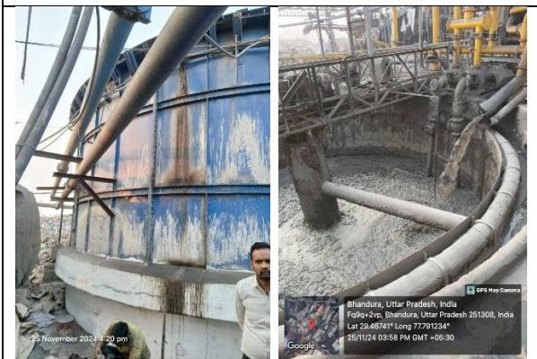
Photo 3: Sedicell & Primary Clarifier
