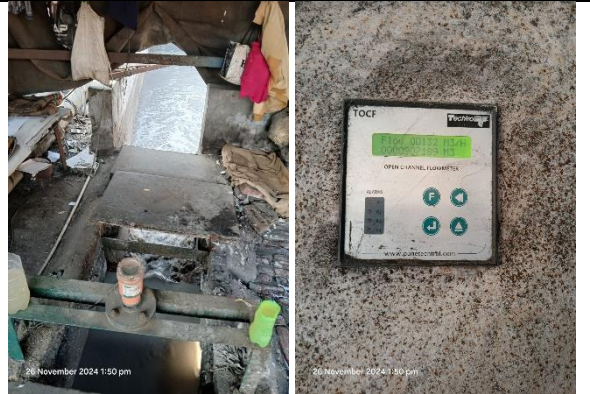
Photo 2: ETP & Inlet ultrasonic flow meter
