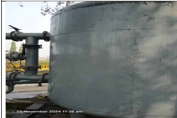
Photo 7: Tertiary filtration system
