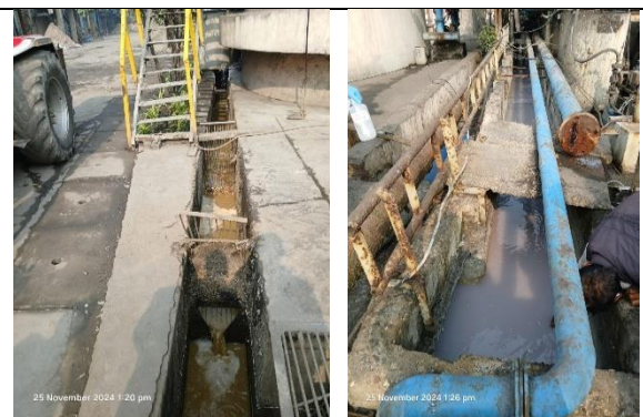
Photo 2: ETP inlet (unit-1 & 2)
