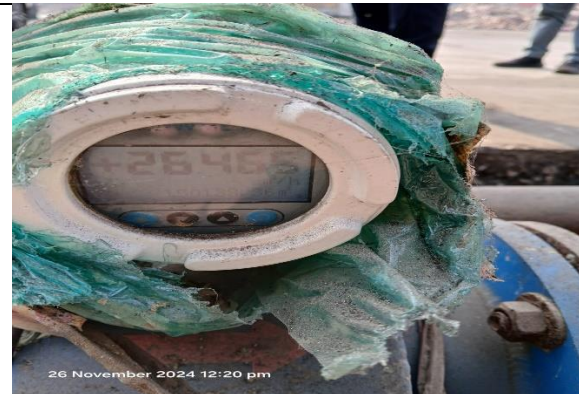
Photo 5: Flow meter on common line carrying Sedicell fiber & primary sludge from both ETPs
