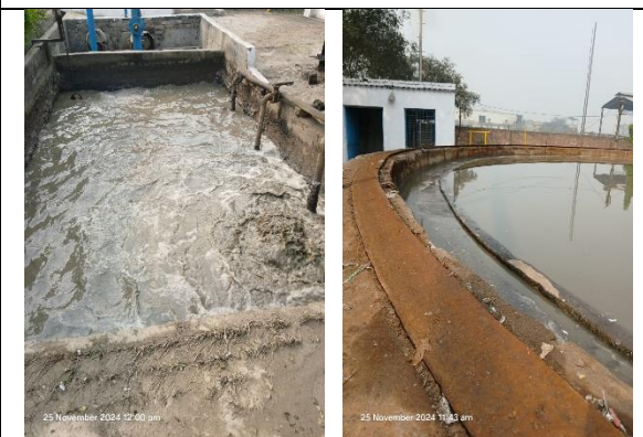
Photo 4: Equalization tank & Primary Clarifier
