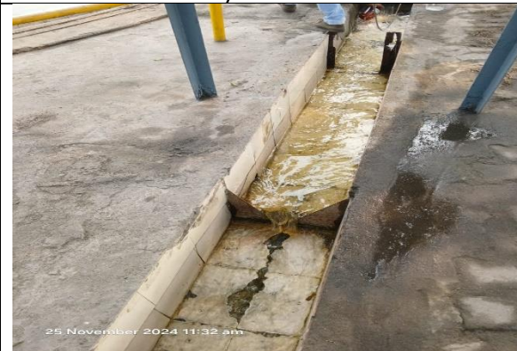
Photo 8: ETP outlet channel
