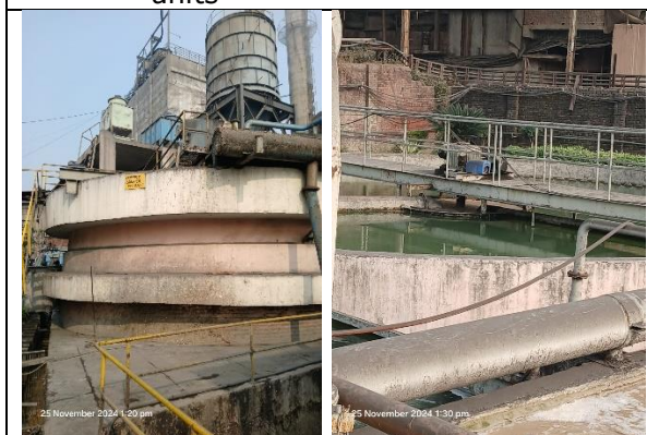
Photo 3: Primary Clarifier (Unit-1 & 2)
